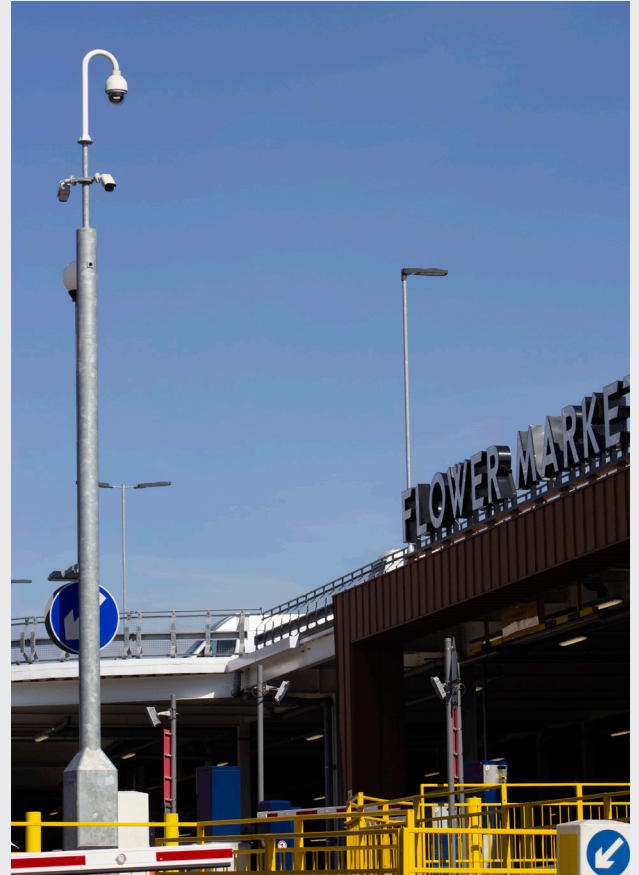
The FLIR bullet and PTZ cameras at New Covent Garden Market provide wide area coverage, along with a greater level of image quality and detail than the market’s previous security system.
